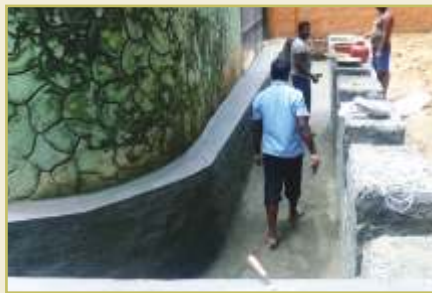
Drain at Neelghai Enclosure: Whenever there is heavy rain due to improper drainage water stagnation at the end of Neelgai enclosure is used to be a common problem. The drainage was constructed to facilitate the flow of rain water & the problem was resolved.
