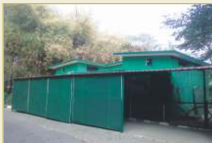
Snake enclosure: Improvements done to Anaconda enclosure and also Provided with Yelahanka tiles over Anaconda enclosure
