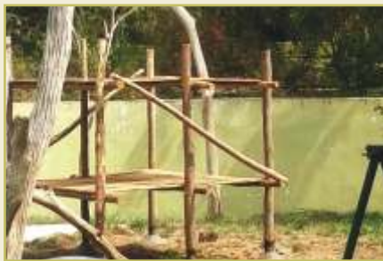
Enrichment Work at Chimpanzee Enclosure: A raised platforms along with swings were installed as an enrichment for the chimps. The animals utilize these things in a proper manner.
